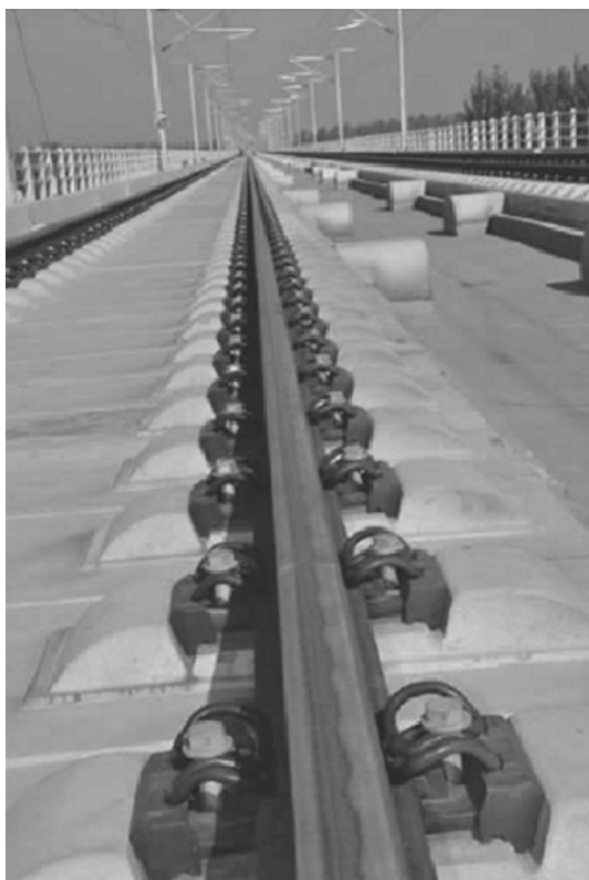
Fig. 1 Rail corrugation in a high-speed track [27]
