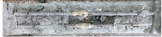
FIGURE 3: Tensile rebar in beam specimen B7.
