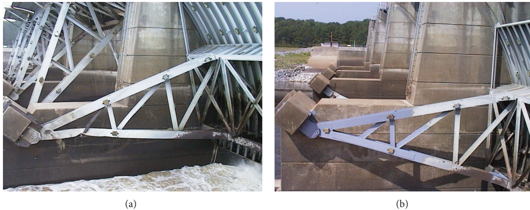
FIGURE 5: Tainter gate with strut arm damage from barge impact before and after repairs.
