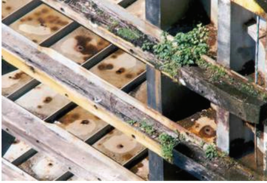
FIGURE 1: Corrosion on a miter gate.
