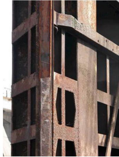
FIGURE 3: Quoin block failure.
