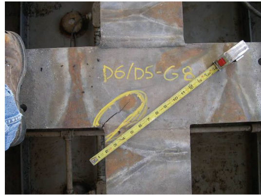
FIGURE 7: Fatigue crack in girder flanges of miter gate.
