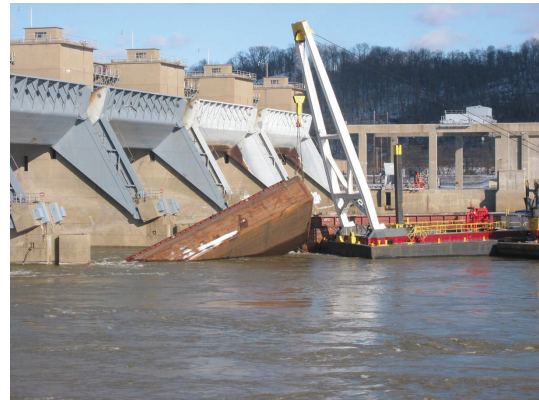
FIGURE 4: Barge impact at Belleville Locks and Dam.
