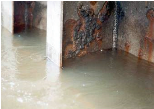
FIGURE 2: Corrosion inside a lock miter gate compartment.
