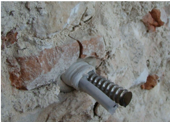
Fig. 6 Typical masonry failure mode during pull-out tests
