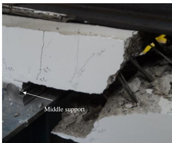
Figure 3–12: Flexure–shear failure at middle support of slab C–B–UO
