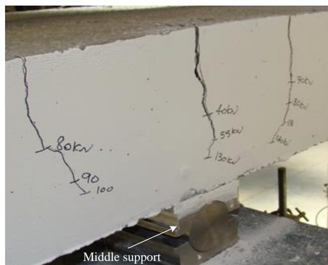
Figure 3-17 : Flexural-tension failure at middle support of slab C-S-UU
