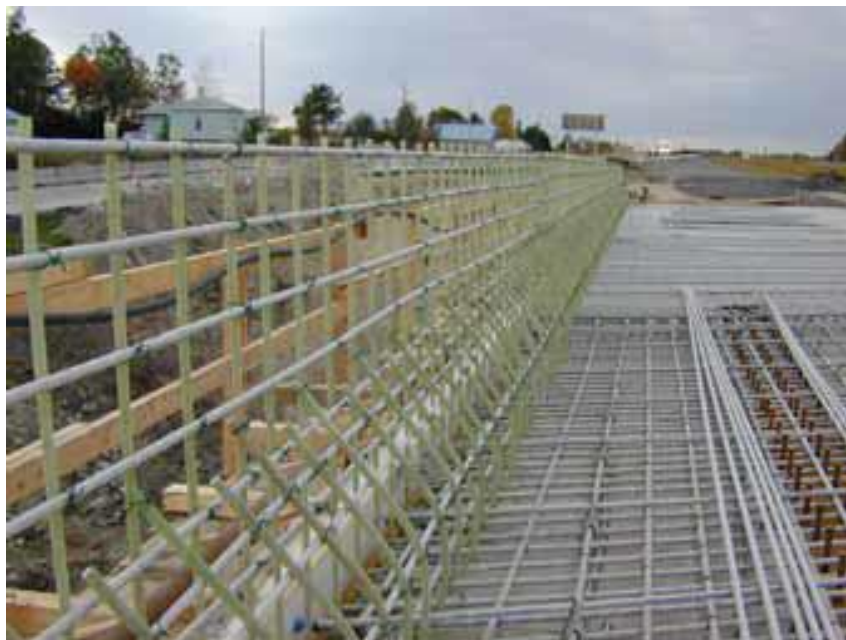
Figure 2–1: Application of FRP as reinforcement in civil and structural engineering (Val-Alain Bridge)
