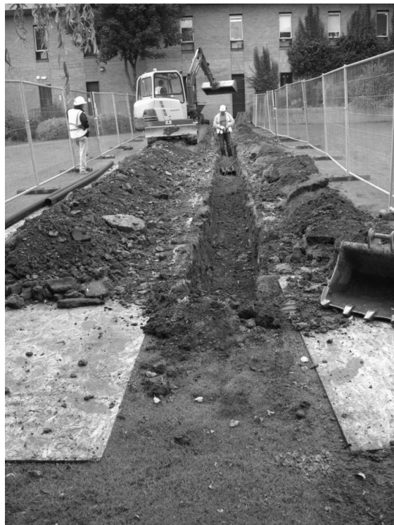
Figure 4.13 The piping for the cabling being laid before sand was added then finally levelled with the previously excavated material.
