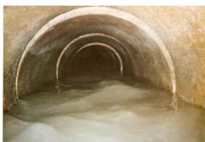
(7) Heavy joint displacement, lightly slimed, clayware pipe, 450mm diameter, k_s^r = 6\text{mm} .
