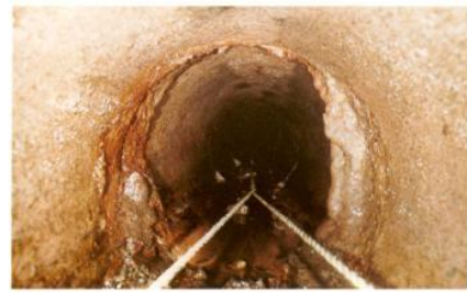
(10) Heavy encrustation at joints, medium debris, clayware pipe, 225mm diameter, k_s^r = 15\text{mm} .
