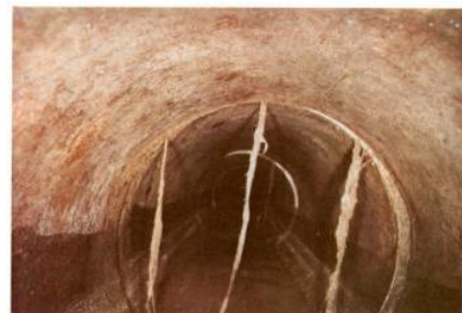
(4) Slight joint displacement, fine roots penetrating joint gaps, slimed to 1/3 depth snup, concrete pipe, 450mm diameter, k_s^r = 3\text{mm} .
