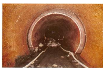
(8) Open joints, joint displacement, debris on invert 5% loss of diameter, clayware pipe, 305mm diameter, k_s^r = 6\text{mm} .
