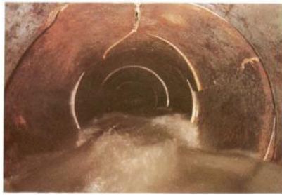
(11) Longitudinal cracks, broken pipe pieces, heavy joint displacement, clayware pipe, 450mm diameter, k_s^r = 15\text{mm} .
