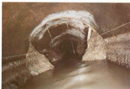
(13) Longitudinal cracks, medium encrustation, root penetration, clayware pipe, 305mm diameter, k_s^r = 15\text{mm} .
