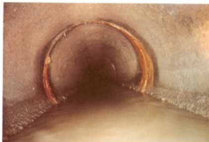
(3) Infiltration at joint, minor encrustation, light to moderate sliming spun, concrete pipe, 600mm diameter, k_s^r = 2.4\text{mm} .
