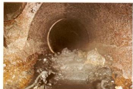
(14) Loss of 15% of cross section, concrete pipe, 305mm diameter, k_s^r = 15\text{mm} .
