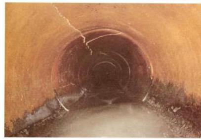
(2) Slight joint displacement, lightly slimed to 1/3 depth, clayware pipe, 525mm diameter, k_s^r = 1.5\text{mm} .
