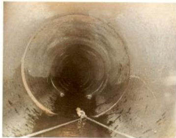
(1) Slight joint displacement free of slime and slit snup concrete pipe, 525mm diameter, k_s^r = 0.3\text{mm} .
