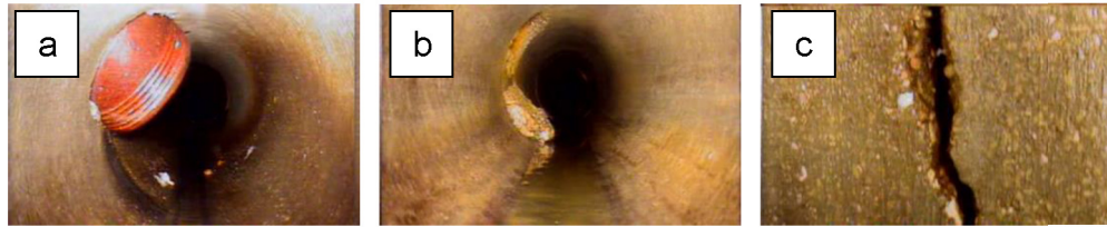
Figure 5.4 Images of sewer conditions recorded by the CCTV: protruding pipe connection (a), hard compacted solid or obstruction (b) and wall crack (c).
