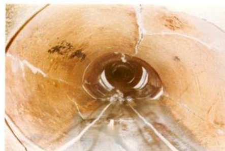
(16) Loss of 25% of cross section, broken pipe, concrete pipe, 450mm diameter, k_s^r = 150\text{mm} .
