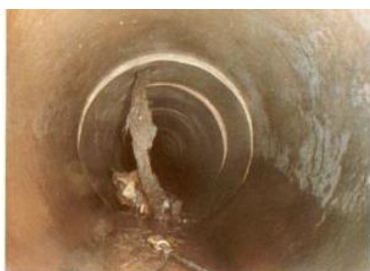
(5) Moderate joint displacement, lightly slimed, blockage, 450mm diameter, k_s^r = 4\text{mm} .
