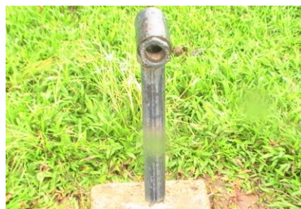
Tap water supply at Bori village
