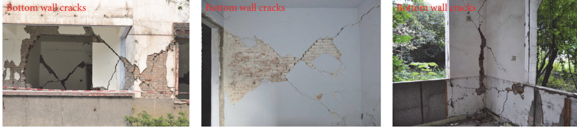
FIGURE 1: Damage of bottom masonry walls during the 2008 Wenchuan earthquake.
