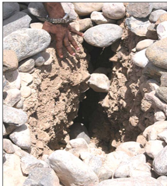
Figure 5. Crack in the crest of the dam at chainage 2+700.
