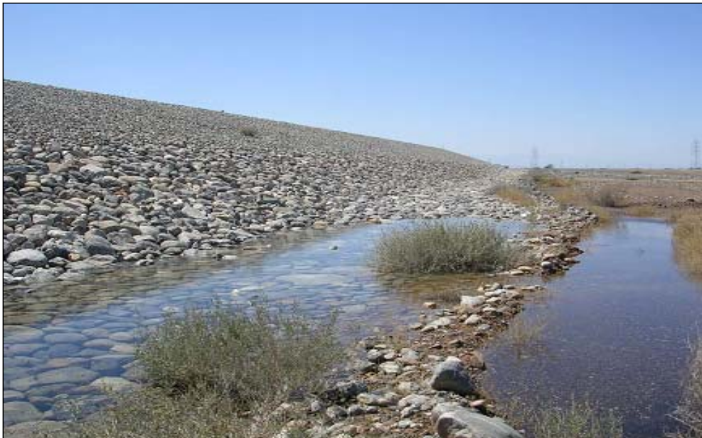
Figure 3. Seepage from the dam.
