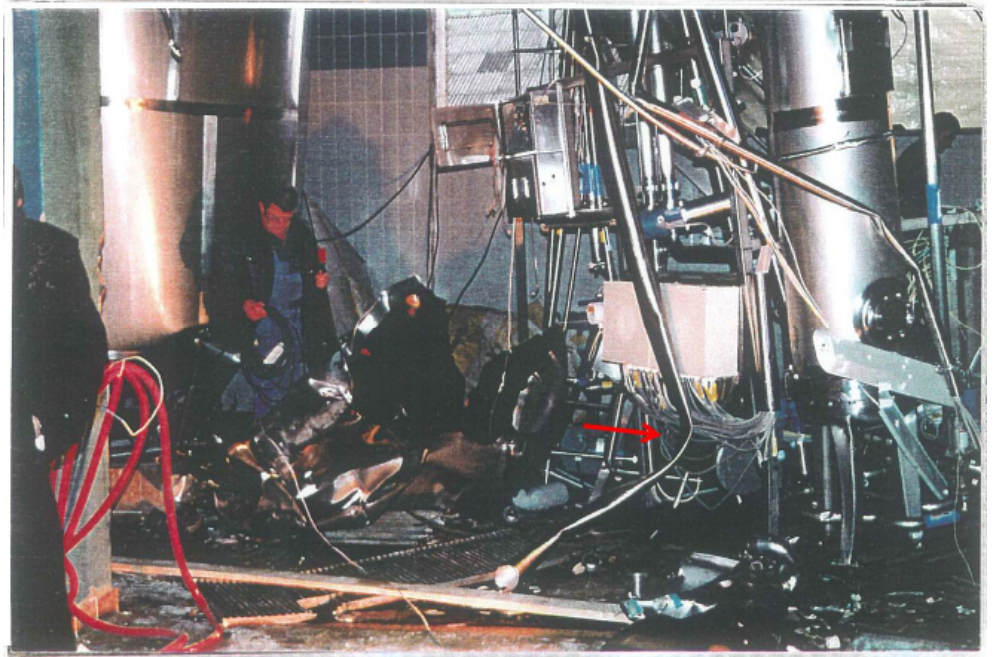
Figure 2 Right: damaged filter unit, left: caustic tank. Note flattened steel piping (arrow). Photo courtesy of company.
