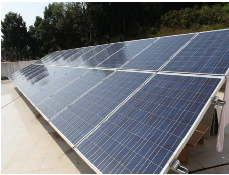
FIGURE 4: The solar panels of solar photovoltaic systems in West Lushan highway service area.
