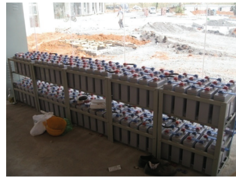
FIGURE 6: Solar photovoltaic power generation storage batteries of solar photovoltaic systems in West Lushan highway service area.
