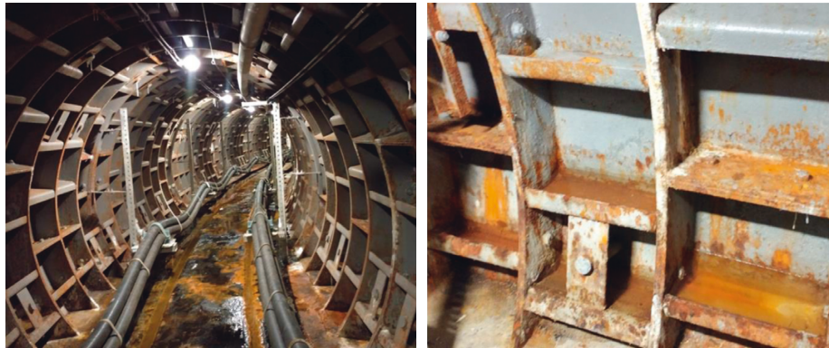
FIGURE 1: Corrosion of steel segments.
