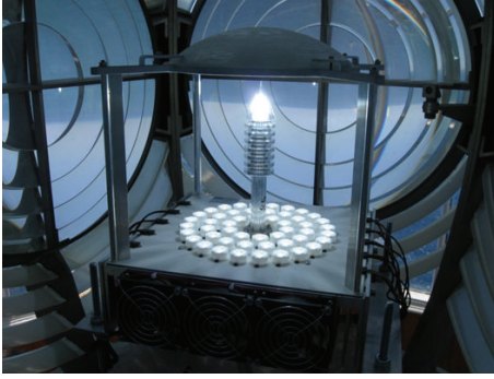
FIGURE 5: New source placed in the lighthouse, 3/4 view from above.
