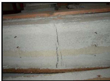
Figure 7 Crack Pattern in Composite Beam 2 and 3
