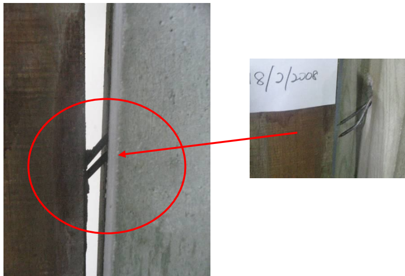
Figure 7. Failure Mode of shear connector with nail
