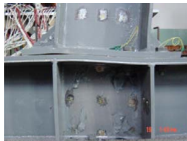
Figure 2.25: Failure mode for EPC-1
