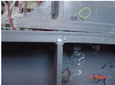
Figure 2.28: Failure mode for EPC-2
