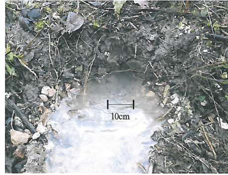
FIGURE 6: 10 cm diameter resurgence observed at the foot of the downstream slope.
