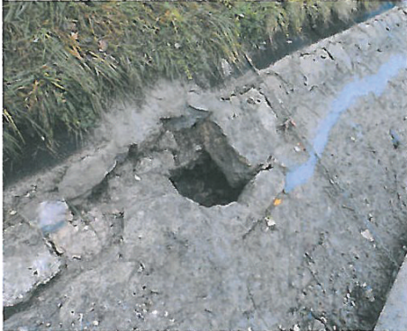
FIGURE 5: Example of serious undermining by internal erosion in the upper part of the paved revetment.
