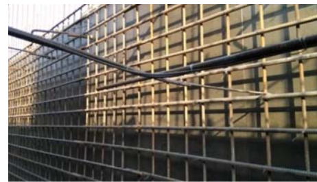
FIGURE 10: The optical cable fastened in the middle plane of the concrete block.
