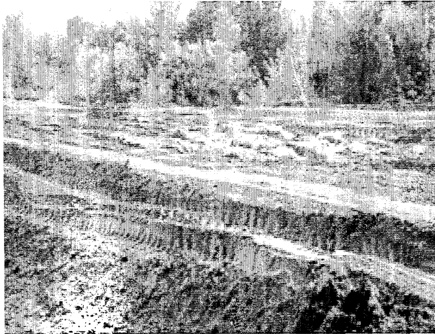
FIGURE 20 Unstable embankment of A-2-4 material
