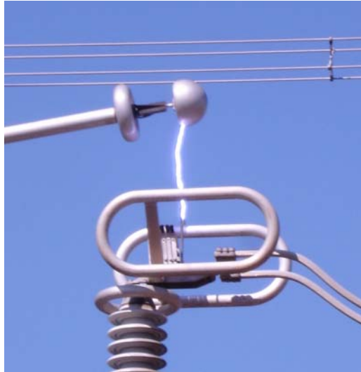
Figure 2. Arc present in the air disconnect switch during an operation.
