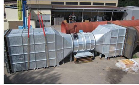
FIGURE 11: The first production Marmaray 2.8 metre two-stage double ended motor fan, transform, silencer, and damper package set up prior to its aerodynamic and acoustic test.
