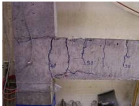
(c) Cracks at region C
