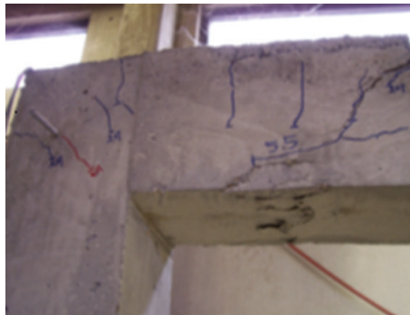
(a) Cracks at region A
