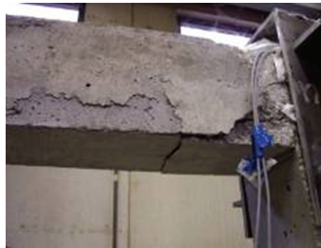
(b) Cracks at region B
