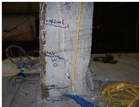
(e) Cracks at region E
