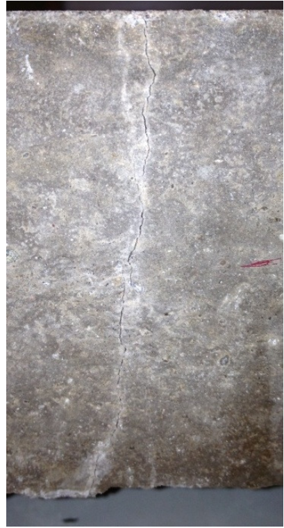
(b) formation of a crack at centre of beam
