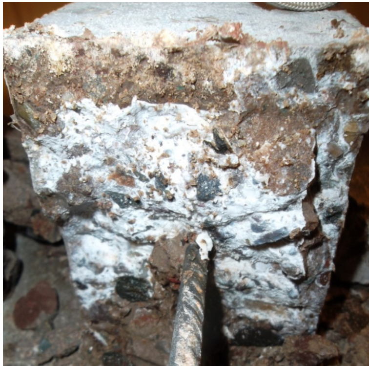
FIGURE 6.8 MINERAL DEPOSITS THROUGHOUT THE CRACK IN BEAM D2
