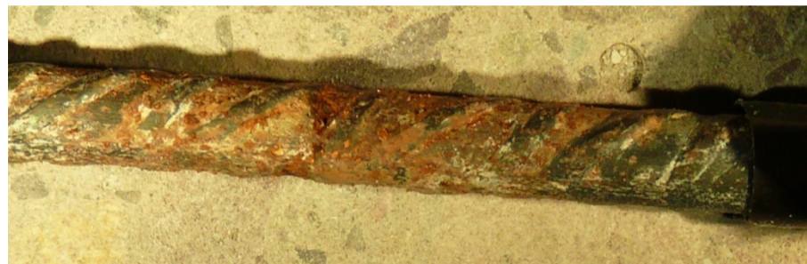
FIGURE 6.13 CORROSION OF 40MM REINFORCEMENT FROM BEAM D2 (0.7MM CRACK WIDTH) AFTER 180 DAYS EXPOSURE
