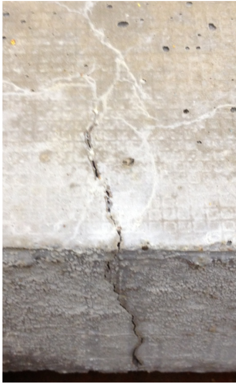
a) 0.7mm crack in seawater
