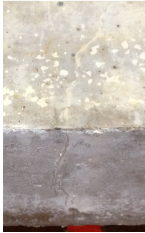
b) 0.2mm crack in seawater
