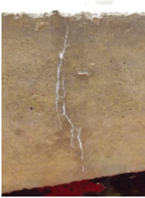
a) sealed crack (seawater)
