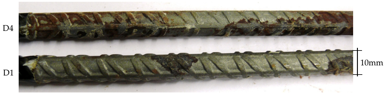
FIGURE 5.15 VARIATION IN PROPORTION OF POLARIZED ANODIC AREAS IN BEAMS D4 (TOP) AND D1
