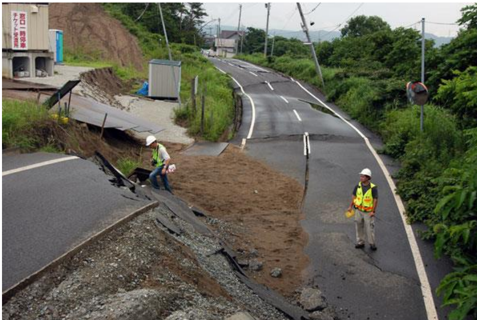
Figure (1- 3): Landslide observation by USGS team (USGS webpage)
