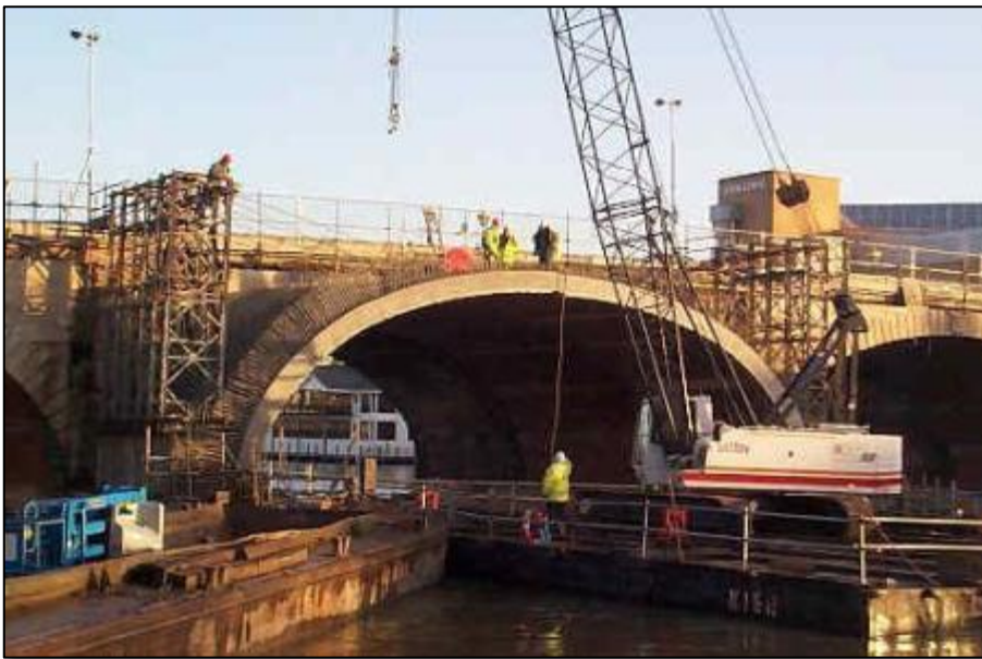
Figure 7.1: Widening and strengthening of Kingston Bridge, West London ( http://www.lobeg.com/index.php?option=com_content&view=article&id=5&Itemid=13 , November 2010)
