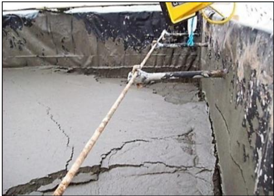
Figure 7.4: Collapsed foamed concrete in Gerrards Cross project
