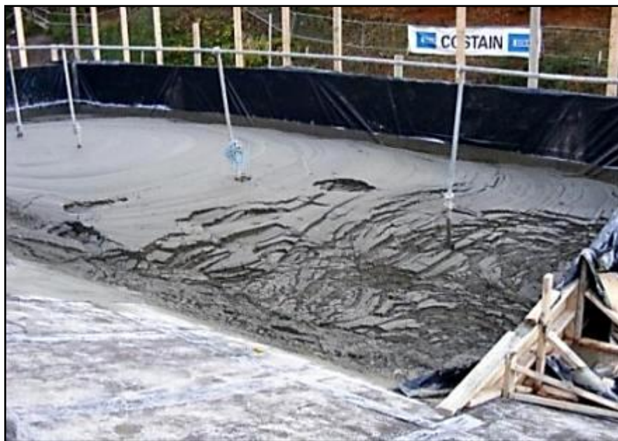
Figure 1.3: Collapsed foamed concrete in Gerrards Cross project (Courtesy of Propump Engineering, Ltd 2010)
