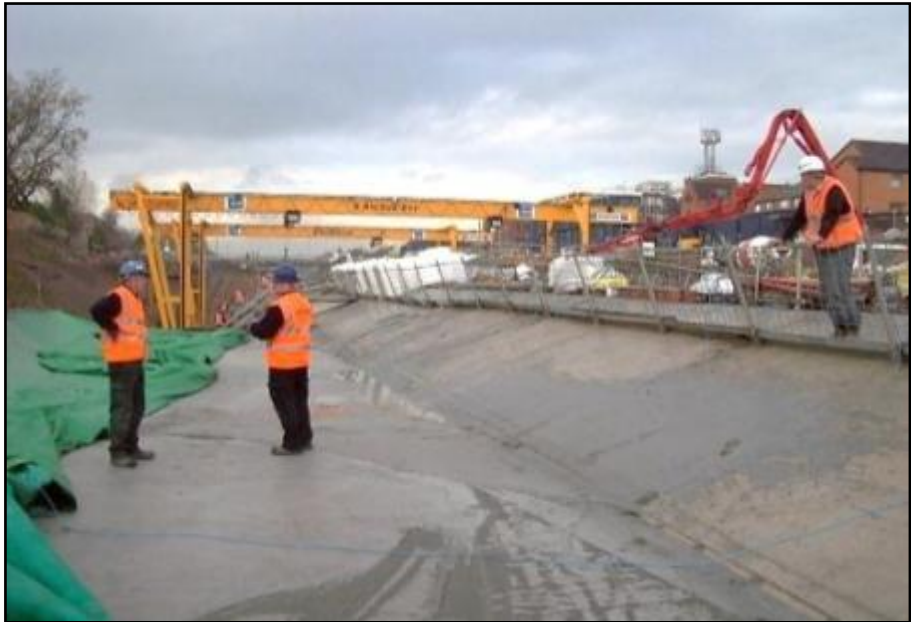
Figure 7.3: Stable foamed concrete in Gerrards Cross project (Courtesy of Propump Engineering Ltd, UK)
