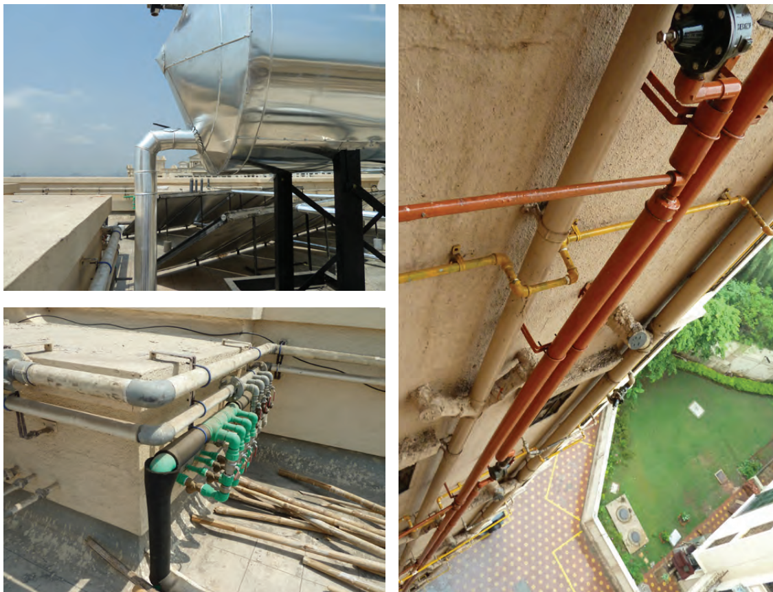
Figures 6.13, 6.14 and 6.15: Material relations: water outlet from hot water storage tank to collector (top left), and hot water piping linking the SHW systems with each flat (bottom left and right).
