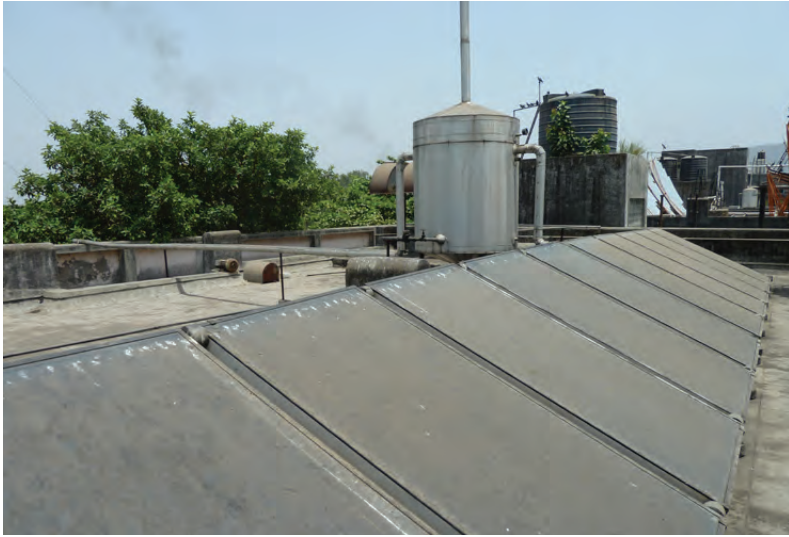
Figure 5.3: SHW systems at Thane's main public hospital.
