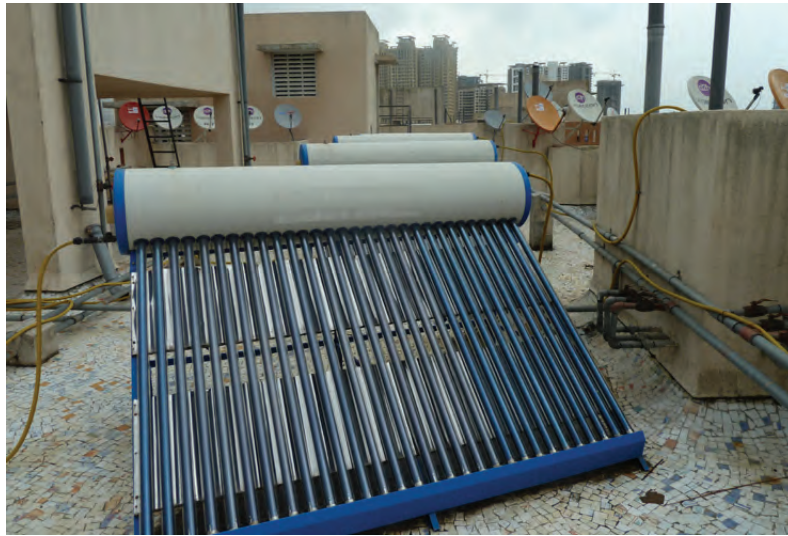
Figure 6.9: SHW system based on evacuated tube technology in Thane.
