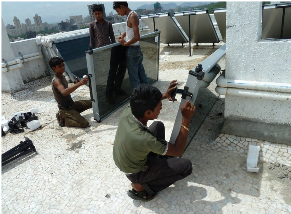
Figure 6.12: Installers of SHW systems, Thane.
