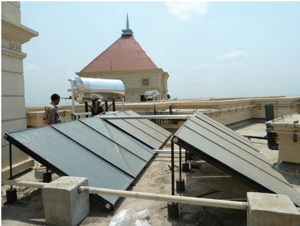
Figures 6.24: SHW at the Gemini Tower (Hiranandani Meadows). The system is composed of 2 tanks and 11 collectors per tank. With 1,300 litres per tank, the system provides 2,600 litres of hot water every day. The tower has 27 stories and 104 flats. The system provides 25 litres per flat.
