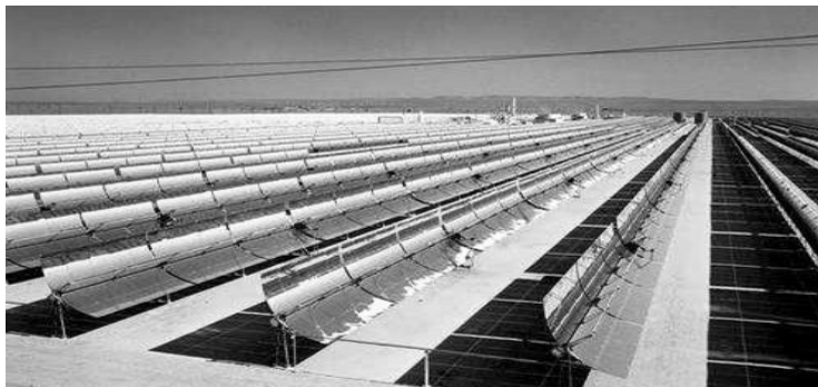
Figure 2.1: A large solar mirror collector field located at Kramer Junction California, USA [14].
