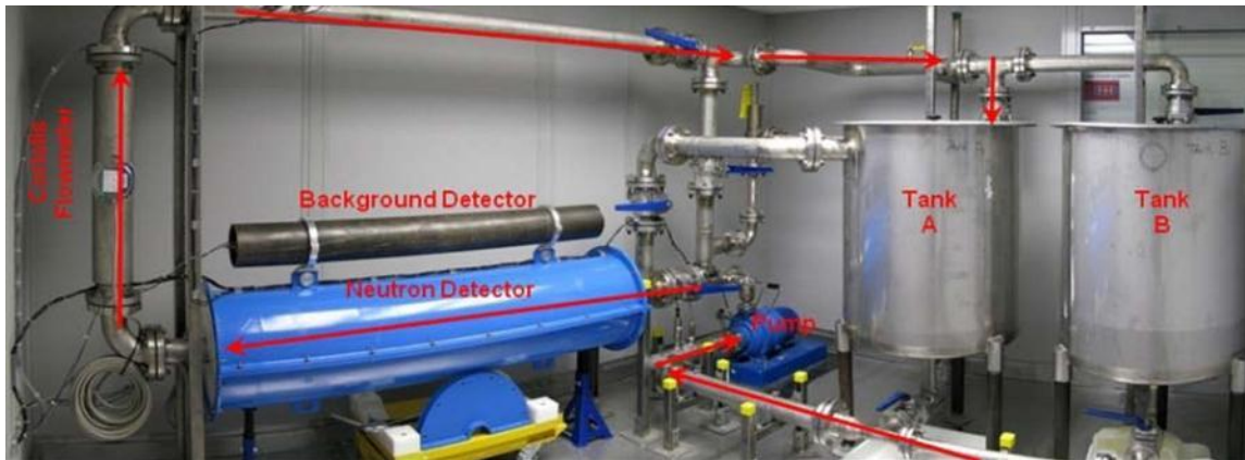
Figure 4-3. UNCLE Facility with First-Generation TUrND Neutron Detector.
