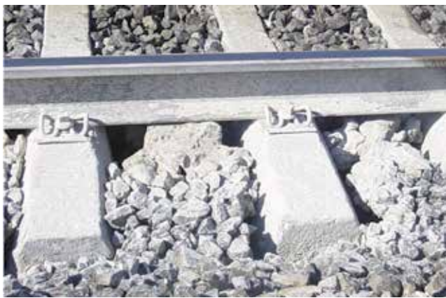
Figure 11. Track surface inspection system – mud & moving sleepers detection
