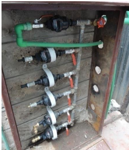
Figure 5-19 Meter bank at Top 1 (Source: Author, 2011)
