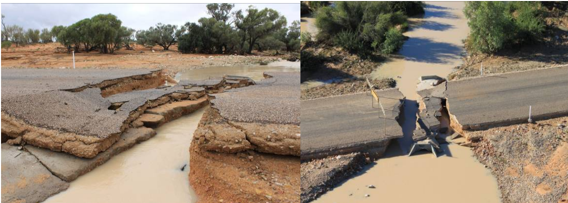
Figure 2. Flood damaged roads in Central West Region, Queensland, Australia in early 2011 (DTMR, 2011)
