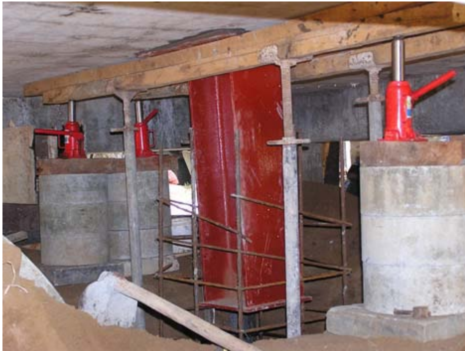
Figure 14: Centre Column H Iron Support Jacked Under the Slab Prior to Concreting.
