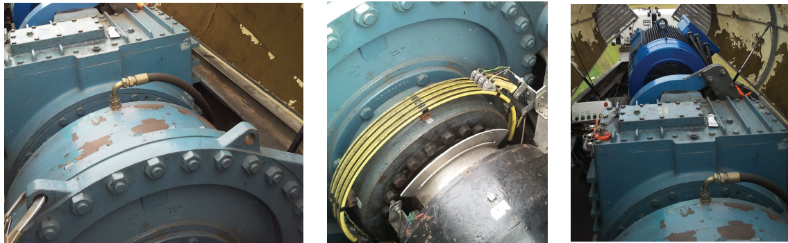
(a) Gearbox (1 planetary gear stage and 2 parallel gear stages). (b) Slip rings on main shaft (gearbox front). (c) Gearbox (front) and generator (back).
