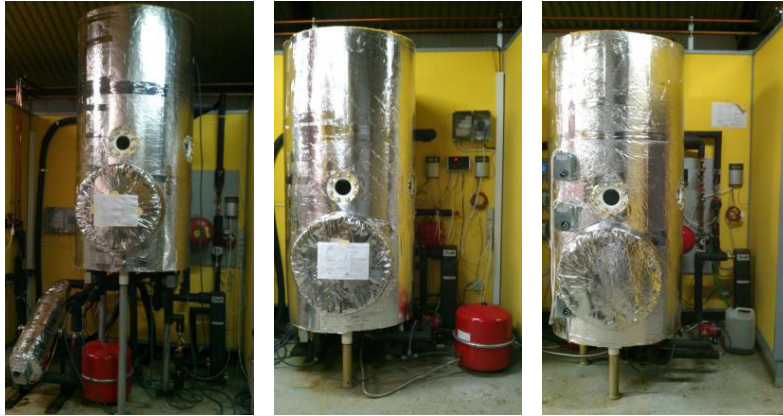
Fig. 2: The heat storages of the three solar heating systems which are being tested.
