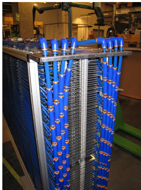
(b) Manifold fittings
