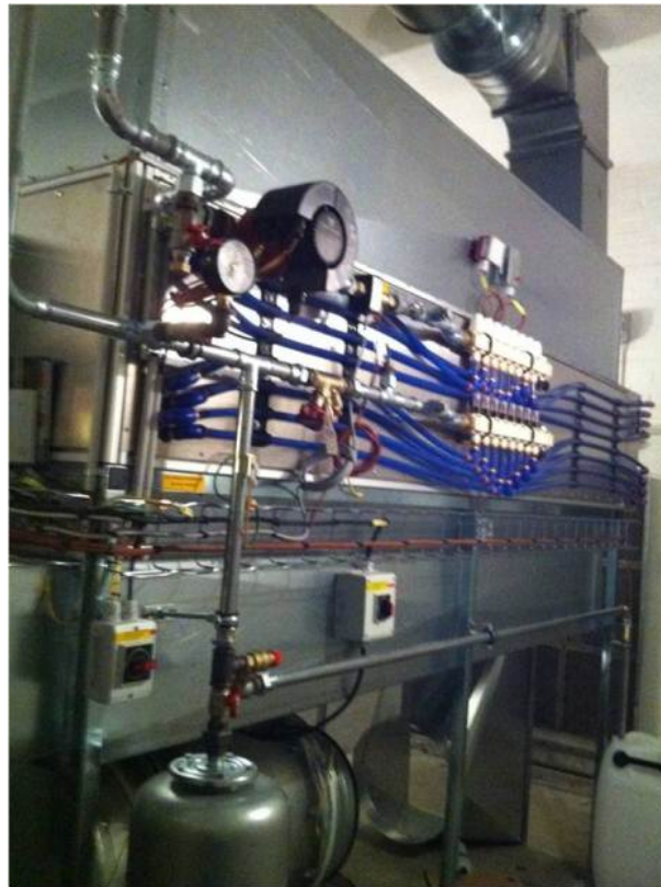
(a) Exchanger coil in the basement
