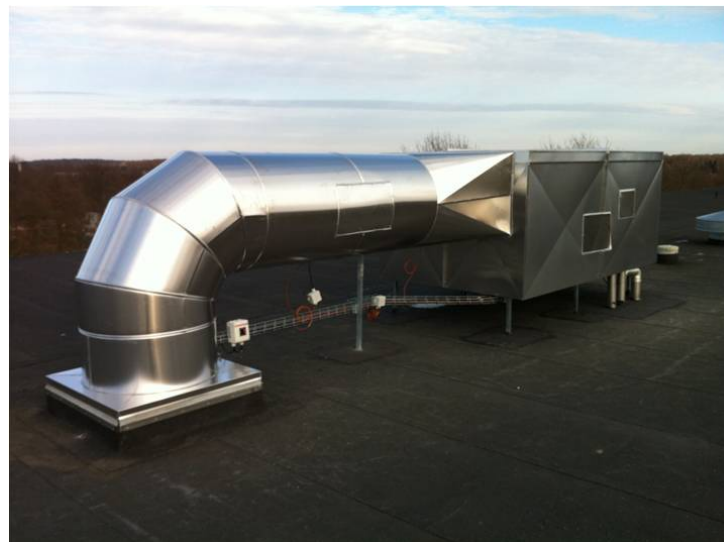
(b) Exchanger coil on the roof
