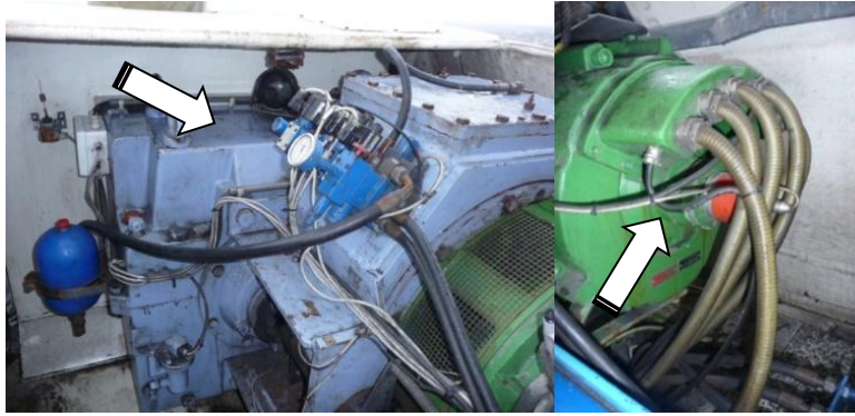
Figure 3a. The position of the accelerometers and the AE sensors for: a. the gearbox and b. the generator.
