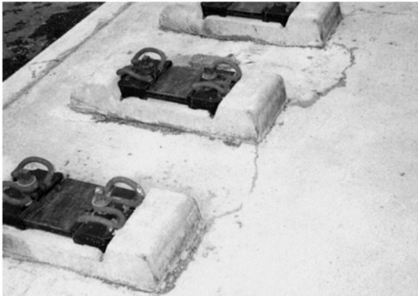
Fig. 2. Problems encountered during use of the concrete ballastless track System
