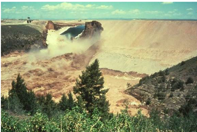
Figure 10. Images of the rupture of the Teton Dam, on the river of the same name, on 5 June 1976, Rexburg, Idaho.
