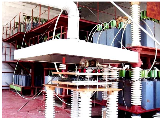
Fig. 1. General view of a powerful high-voltage high-current generator of artificial lightning current of the type УИТОМ-1 (in the foreground there is a desk with a high-voltage three-electrode air controlled switch with steel electrodes for a voltage of \pm 50 kV and pulsed sinusoidal lightning current up to \pm 220 kA, a tested sample of the skin of an aircraft and an air drawing system, and in the background – separate high-voltage pulse current generators for the corresponding current components A, B, C, C^* and D ) [11]
