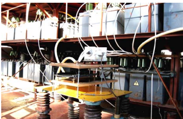
Fig. 9. General view of a powerful high-current generator of artificial lightning current type ГТМ-10/350 (in the foreground there is its working table with placed on top of it a controlled high-voltage three-electrode air switch with graphite electrodes for voltage of \pm 50 kV and pulsed aperiodic lightning current of amplitude up to \pm 220 kA and the tested sample of cable-conductor products, and in the background – the electrical engineering elements of the charge-discharge circuits of its separate high-voltage pulsed current generators PCG-1, PCG-2, PCG-3 and PCG-4) [19]
