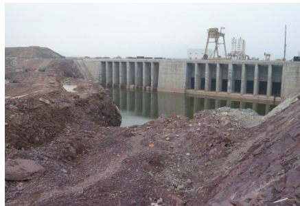
Fig. 2. The blasting site for rock excavation of open channel on land in Taishan
