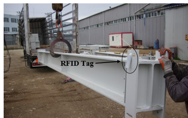
Fig. 4. Steel assembly with an RFID tag
