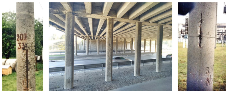
Fig. 1. Circular cross-section reinforced concrete structures damaged by corrosion
