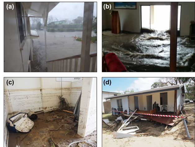
Figure 10. Flooding (a), water ingress (b), interior (c) and exterior (d) damage to property at Wilson Beach. (c) and (d) are authors' own images; (a) and (b) were taken by residents at Wilson Beach, reproduced with their permission for this paper.
