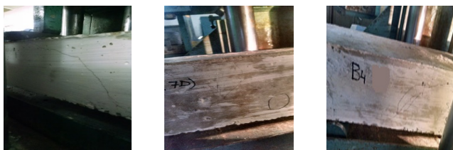
Fig. 4. First crack in beams B1, B3 and B4
