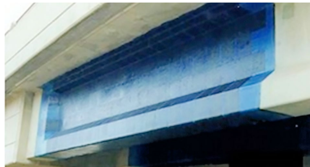
Fig. 5. Externally-bonded carbon FRP sheets for shear strengthening of a reinforced concrete bridge girder (photo from http://www.fhwa.dot.gov/everydaycounts/technology/bridges/pbeswebinartraining/s3_m9.cfm )
