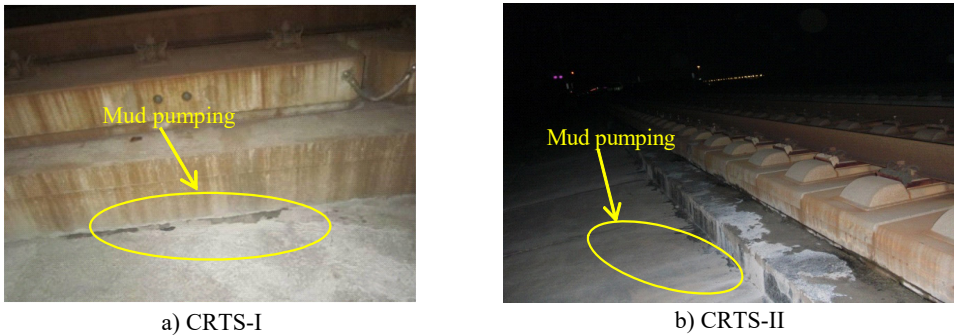
Fig. 1. Example of mud pumping of subgrade surface layer in Chinese high-speed railway
