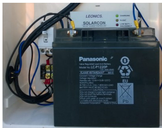
Fig. 7. Battery and charging unit inside the solar charging station.
