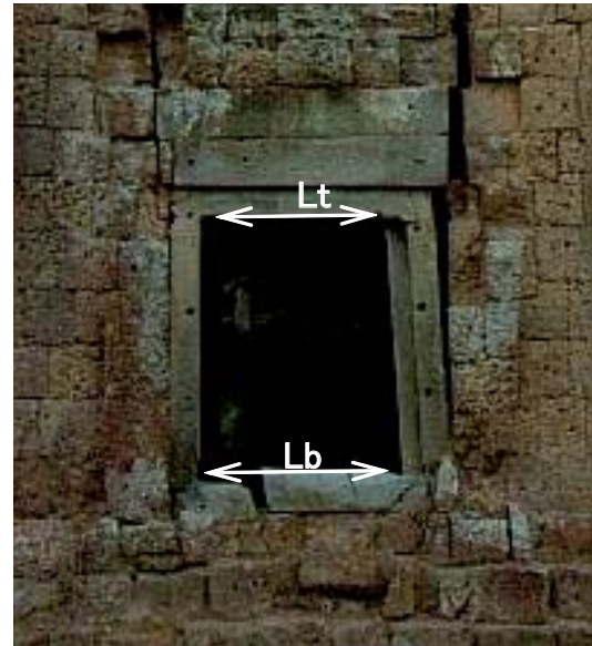
Photo 3. Deformed frame of open window at west side
