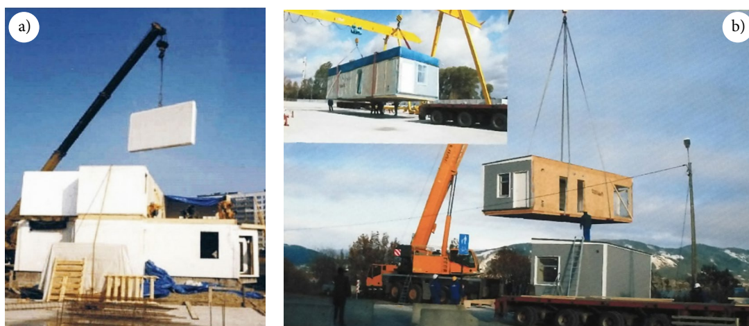
Fig. 10. Assembling of large panel building and module constructed building (Miedziałowski, Malesza 2006; Mohammad 2006)
