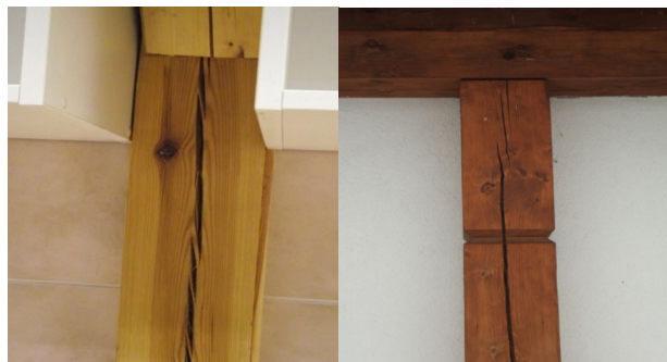
Fig. 18. Supporting post splitting in result of shrinkage
